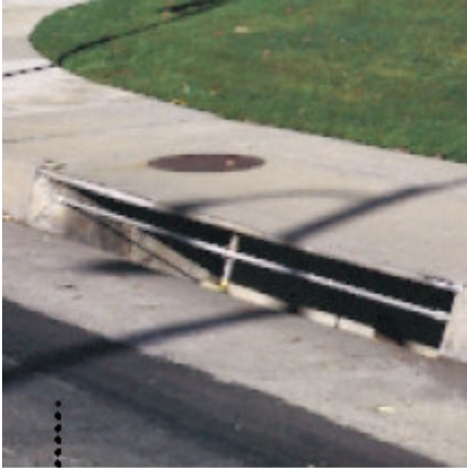
Catch Basins are the major entry points to the storm drain system
